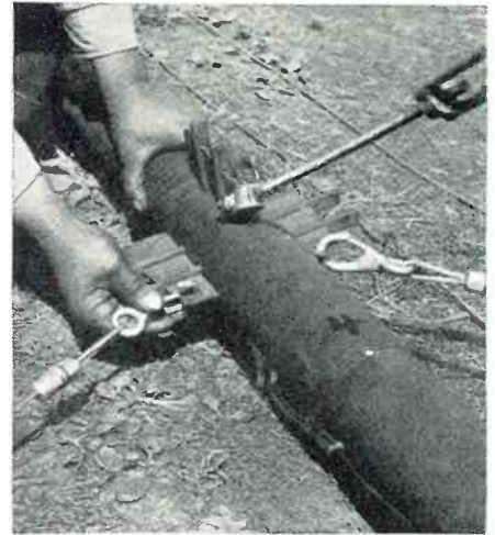
Fig. 1. Wedged bars are used to connect steel pipe sections of radio mast.
