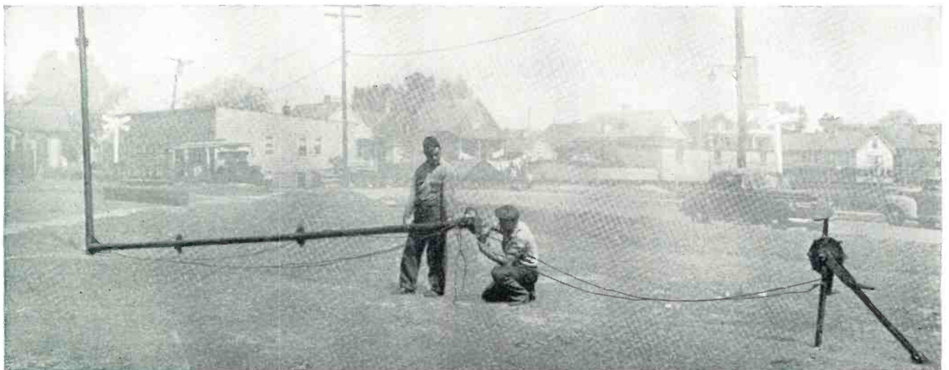
Fig. 4. Winch cable being attached to boom which, in final operation, is used to raise complete assembly into position.
